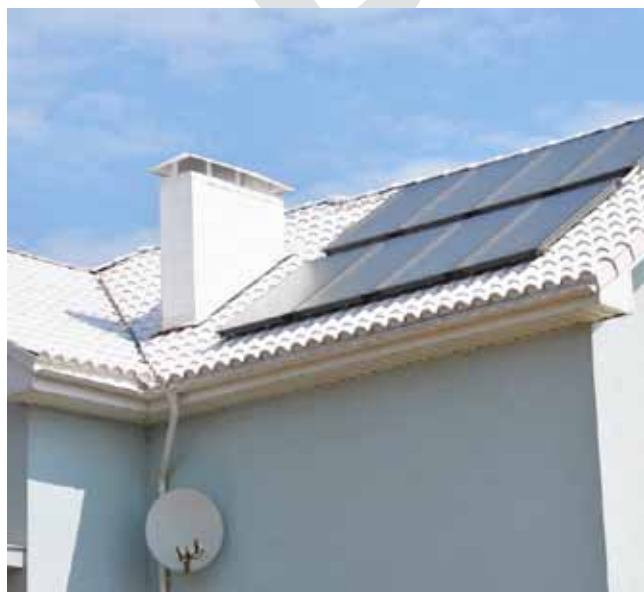
Light-coloured cool roof plus solar PVs
