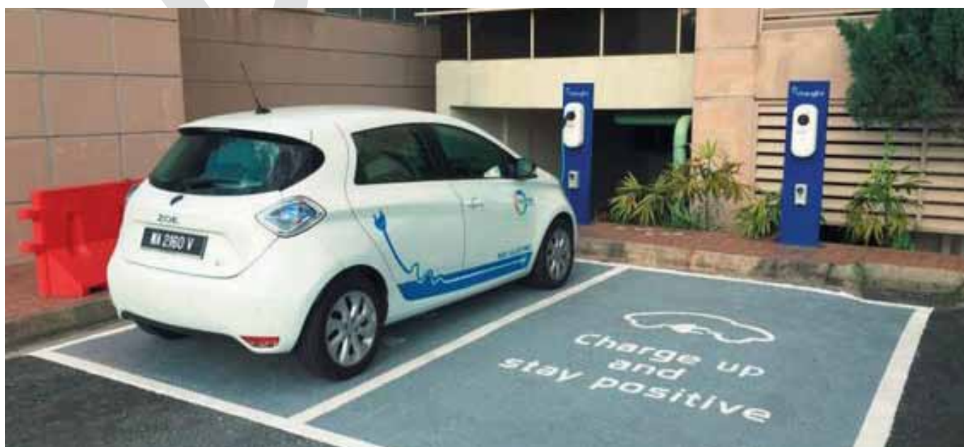
Charging facilities for electric vehicles
