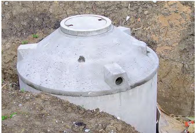
Collect, store and distribute rainwater in underground storage tanks.
