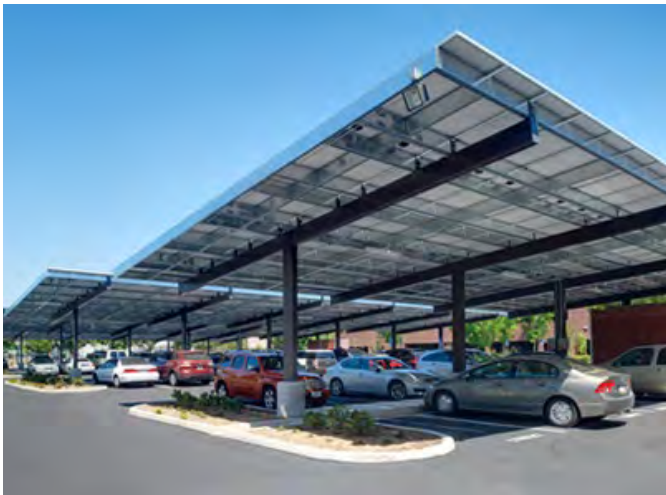
Solar canopies in surface parking lots.
