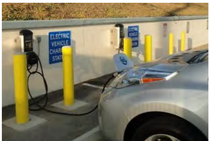
Charging stations for electric vehicles in mixed use areas.
