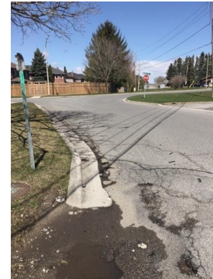
Example of poor road drainage causing damage to the roadway and water ponding
