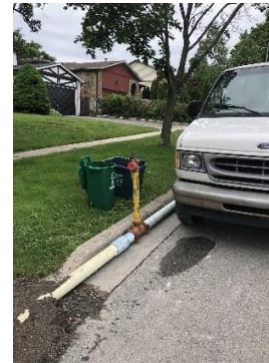
Example of a typical temporary water connection
