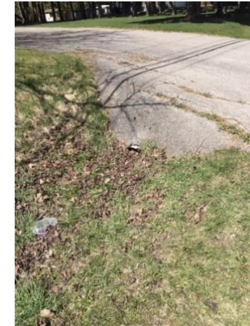
Example of poor pavement condition and partially collapsed culvert
